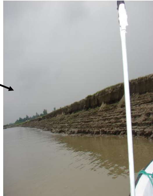
Fig. 3. Eroding river bank before bandals construction
