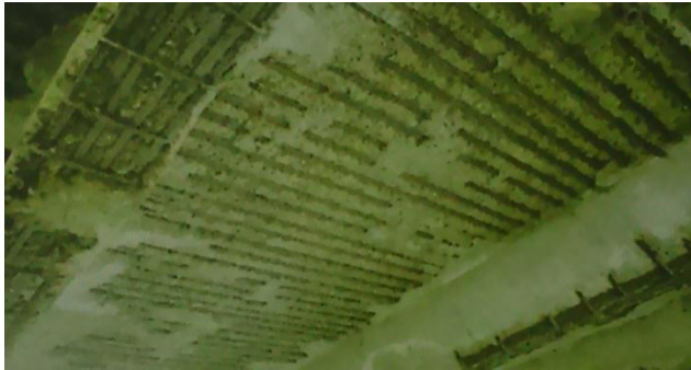
Fig. 1. Corroded reinforcing steel in concrete deck.
